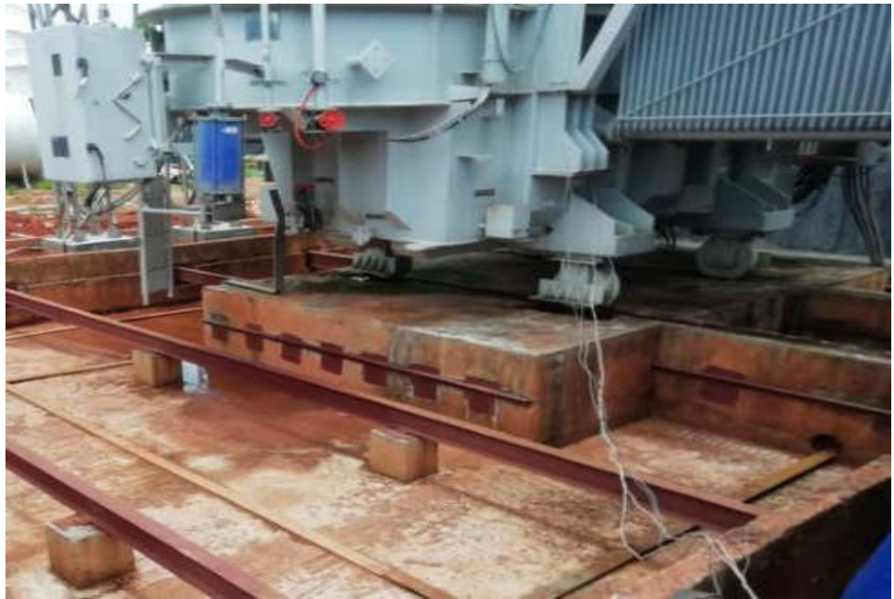
Transformer Oil Sump Pit at Vadakancheri Substation
