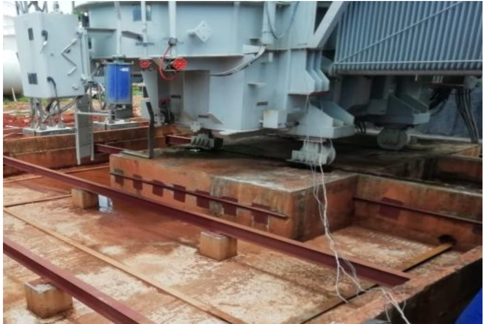
Transformer Oil Sump Pit at Vadamancheri Substation
