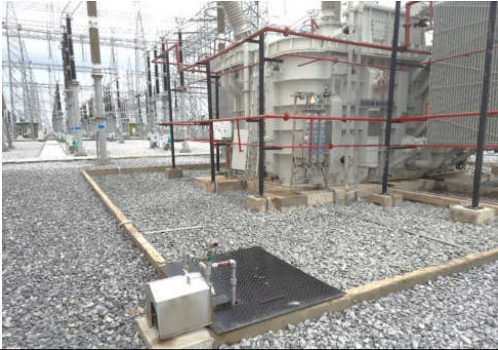
Transformer Sump Substation
