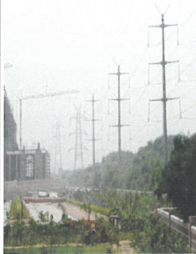
400kV Compact Single Pole Tower
