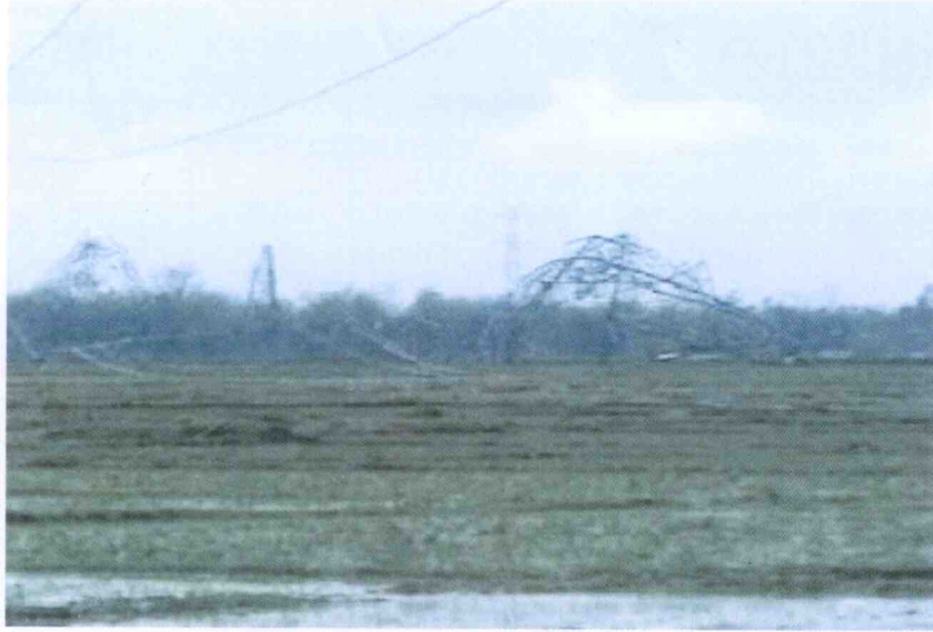
Photograph of collapsed tower
